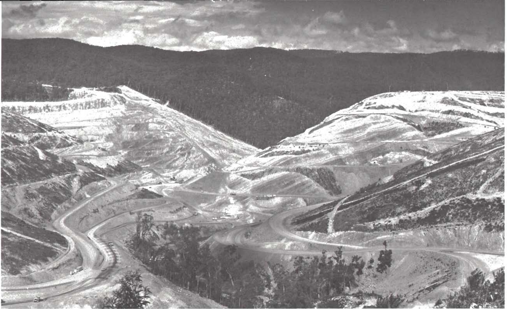
The Thomson River Dam project, north of Erica. When completed, the dam will impound 1,100,000 megalitres of water for supply to Melbourne and for irrigation purposes.
